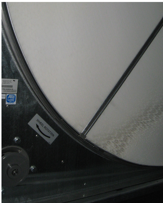
Figure 10: An enthalpy wheel in a central ERV at the Brooks School, North Andover, MA. (Photo credit: Architerra)
