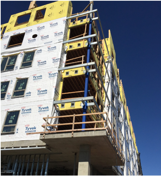
Figure 6: Interior concrete slabs extending unbroken through the thermal envelope and thermally un-broken structural connections turn this multifamily development’s balconies into significant thermal bridges
