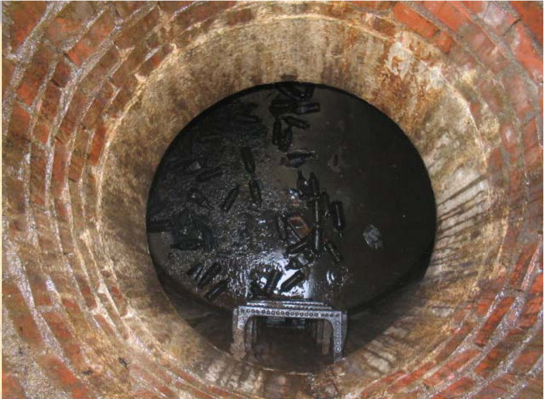
Stormwater BMP in need of service –filled with debris and motor oil- poor house keeping results in the need for frequent maintenance service
