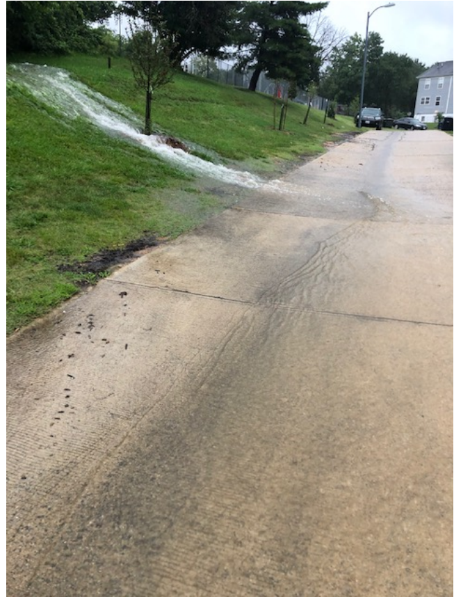
Photo 3: Overflow from Inlet 21
