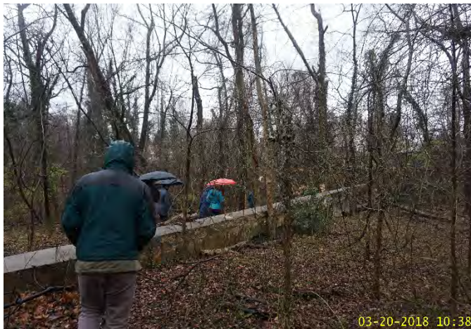
Photo 1 – Above ground sewer line running in a concrete encasement from Branch Avenue to Erie Street.
