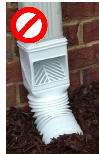
Uncovered filter not permitted
