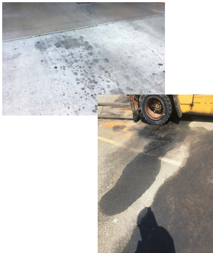
Evidence of Leaks
