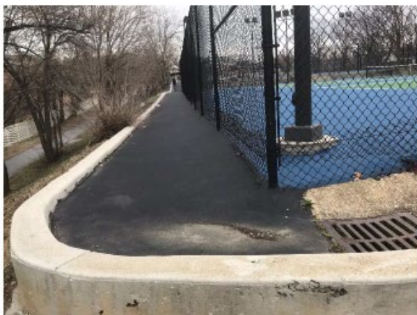
Tennis court curb and inlet
